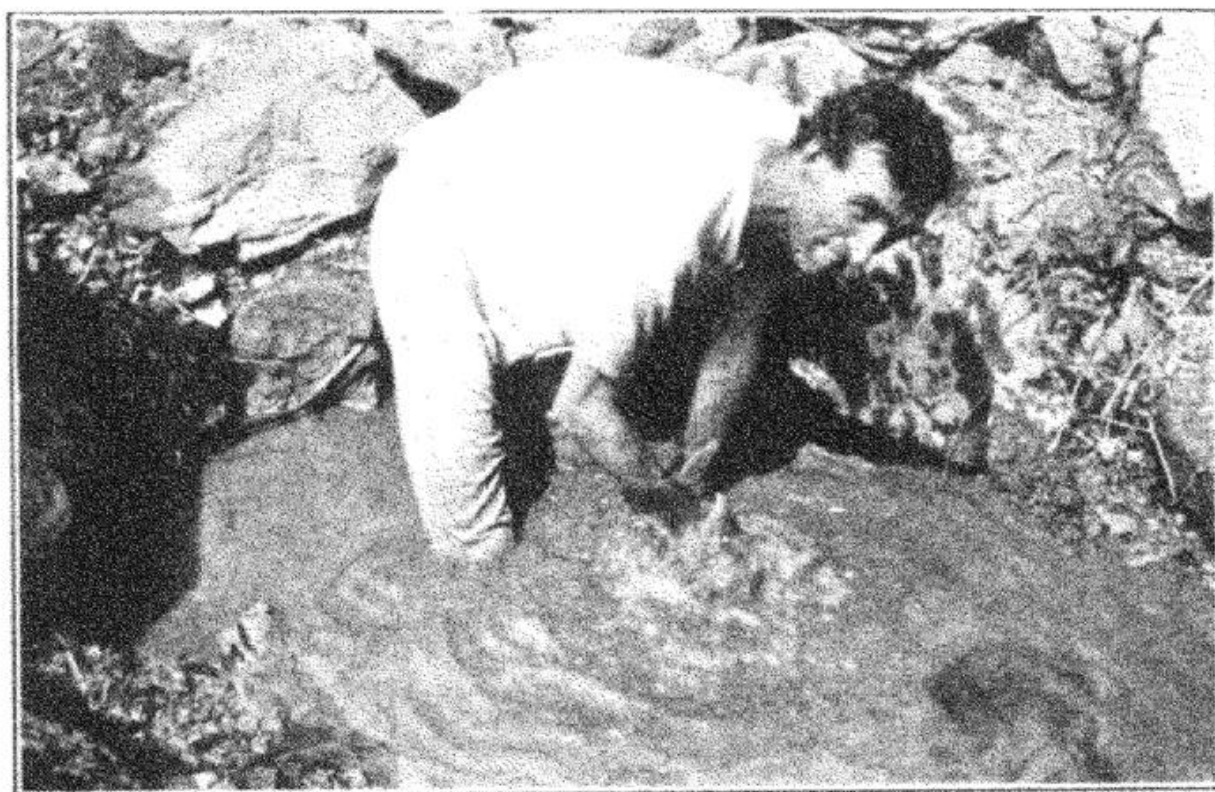
NOT BATHING—REPAIRING A LEAK
