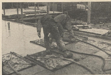
Modern technique dries cement by suction—saves time, saves labor cost. Suction mats at work on Red Hook Project in New York City
