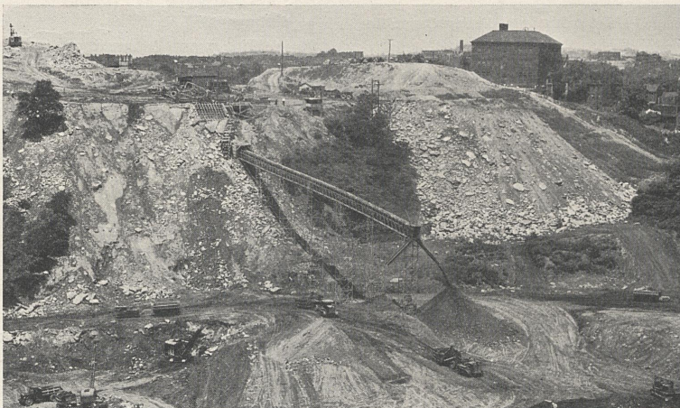
Scarcity of Low-Cost Land Compels Pittsburgh to Level Downtown Hilltops to Provide Project Sites
