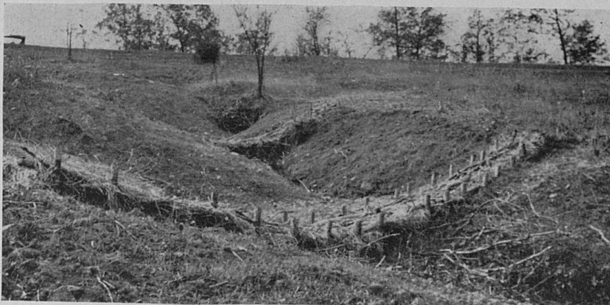
A temporary brush dam constructed across a gully after the sides have been sloped. Quick-growing trees such as black locust are planted in the gully banks to help hold the soil.
