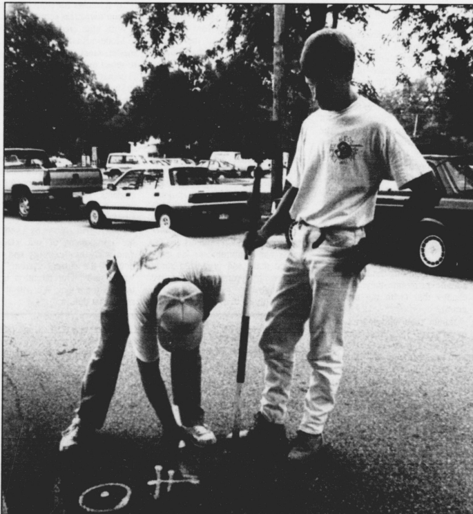
Marking a location on Clifton Circle for a boring sample, Rodman Don Wilkins and Walt Duermit Jr., of FMSM Engineers of Lexington, begin construction on the new library.
