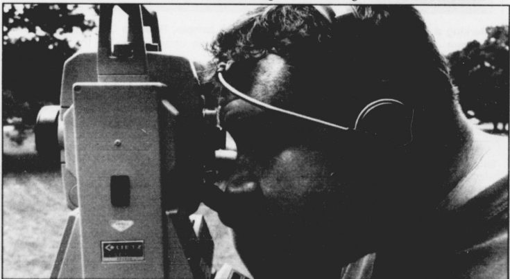
Tom Conlee of FSM Engineers, uses an Electronic Distance Meter to survey various column lines for the new library being built on Clifton Circle. Library construction will continue on the site until the summer of 1996.
