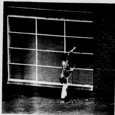
A Physical Plant Division worker removes glass from one of the windows in the Anderson Hall Quadrangle yesterday.
