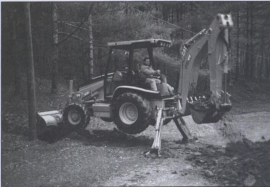
Joey Roberts, Maintenance Foreman, operating the backhoe - replacing drain pipes in Pig Alley
