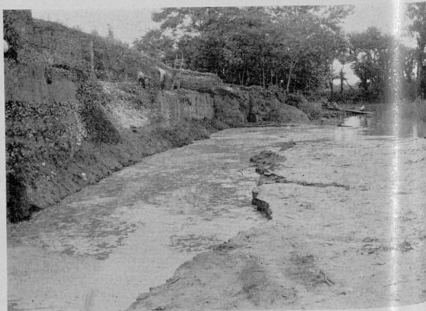
Figure 3. Flood water rising against profile. Earth thrown against profile to prevent cave-in proved ineffective. Looking toward mouth of Flint River.
