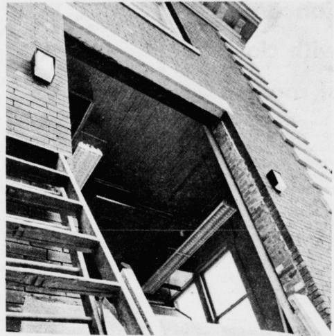
The north wing of Kastle Hall is currently under construction to facilitate a temporary research laboratory for the Kentucky Tobacco and Health Research Institute. (Kernel photo by Phil Groshong.)
