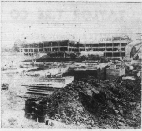
Construction of the power plant for the new Albert B. Chandler Memorial Hospital is shown in the foreground. In the background is the Medical School.
