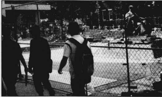
Students walk around the construction taking place in the shadow of the Patterson Office Tower. The work should be completed summer 2004.
