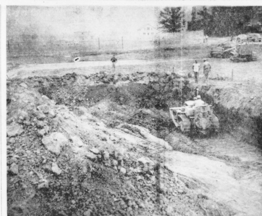
CONSTRUCTION BEGINS ON MEN'S DORM - Excavation started this week on the new men's dormitory to be constructed on Rose Street. It is being built along with five new fraternity houses, and should be finished by next semester.
