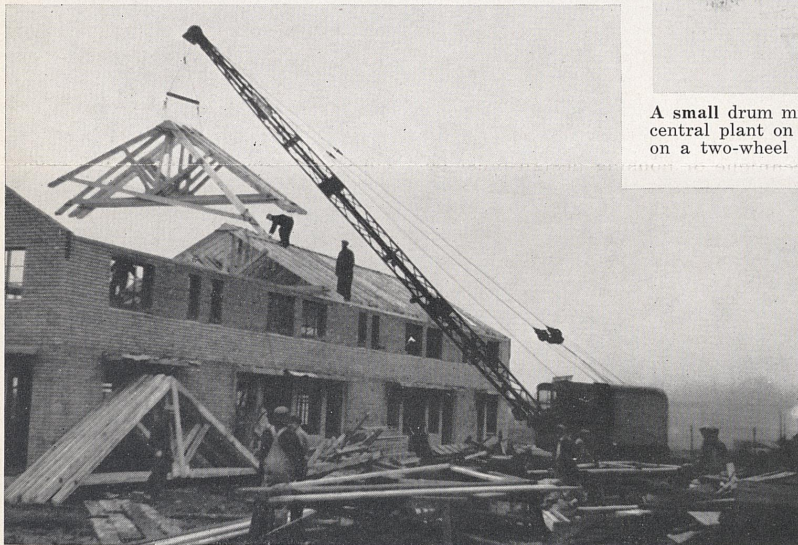
All members of wood trusses for hip roofs were cut and assembled on the ground by use of electric powered saws and templates. After assembly they were raised to position, four at a time, by crawler crane. One carpenter at each end and one at ridge line rapidly placed each truss in position. The crane followed with sheathing after each roof was trussed.
