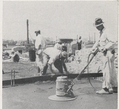
Electric powered finishing machines were used for 433,000 square feet of floors. Electricity was widely used. Poles carried plug boxes for both 110- and 220-volt equipment.
