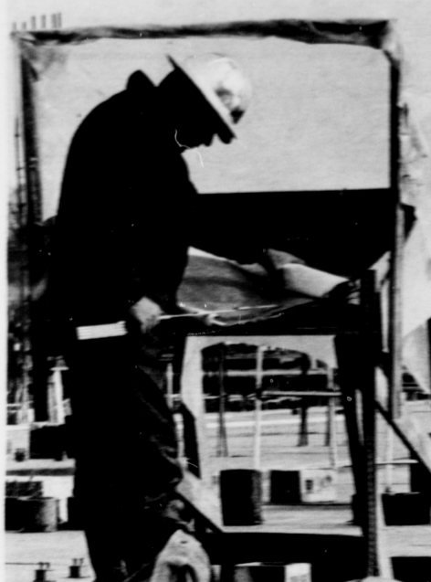
A steel helmeted worker measures specifications on a blueprint. The entire dormitory project under construction will cost $17 million, planners say.
