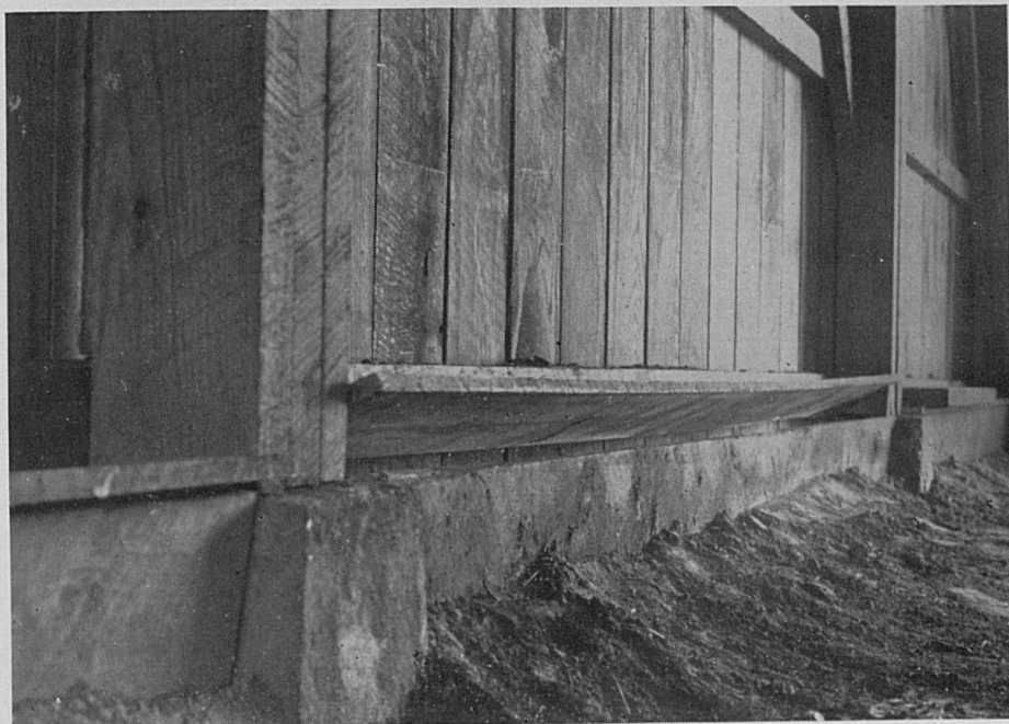
Bottom ventilators built on a fire-curing barn as shown in Fig. 10, between the concrete blocks that support the barn posts. The middle door is shown partially open.
