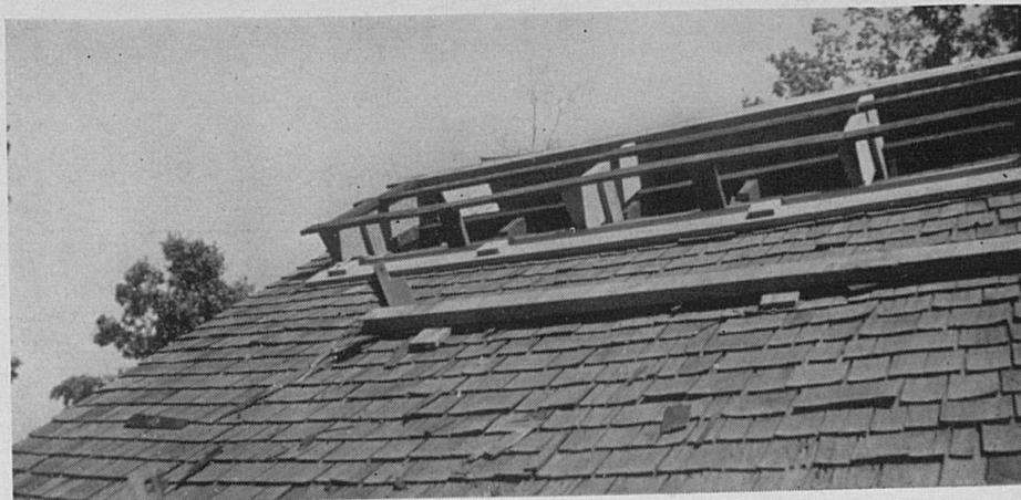
Ridge ventilator being constructed on wooden shingle roof according to Plan No. 1, Fig. 7, page 17.
