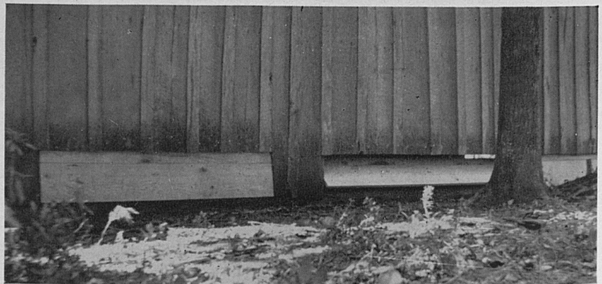
Bottom ventilators built on a fire-curing barn (according to Fig. 11, Page 19) over a solid concrete foundation.
