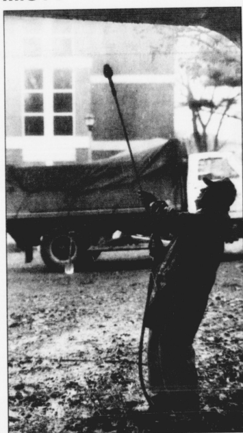
David House, of Cooper and Cooper Painting, pressure washes the underside of the Business and Economics walkway.
